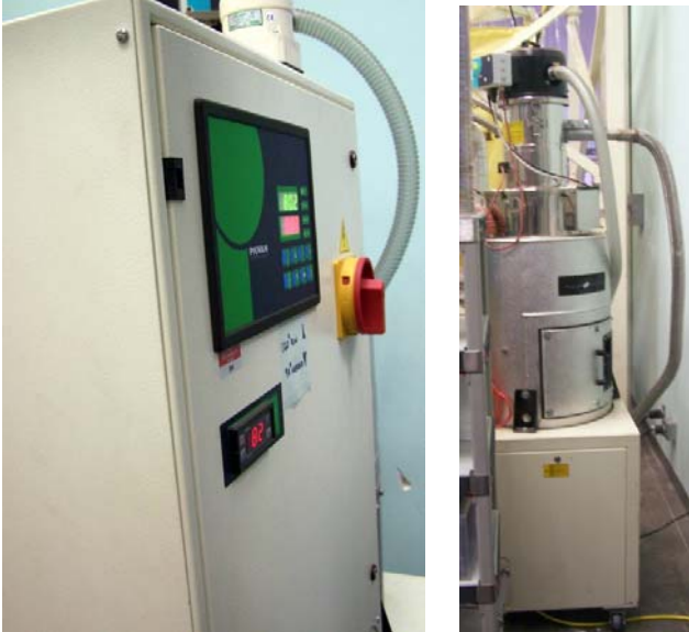
Piovan drying system with dew point monitoring and SS conveying
